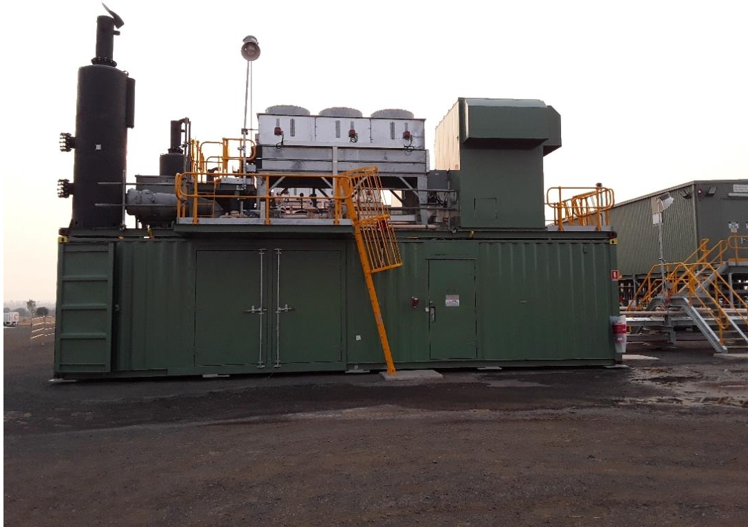
Figure B1: Generator from ACS-02 Site.
