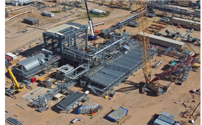
Compressor shelter and heat exchangers
