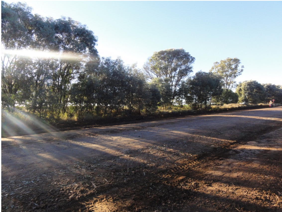
Photo 1.2 Road constructed adjacent to the proposed development area showing patches of Acacia harpophylla (Brigalow) disturbed by recent works
