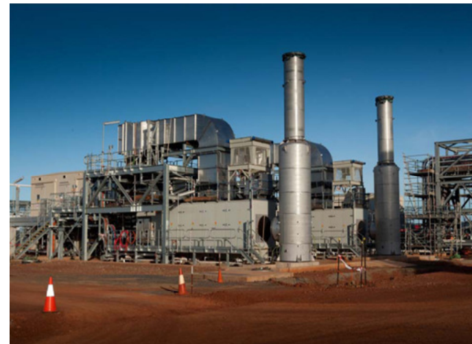
Devil Creek gas plant
