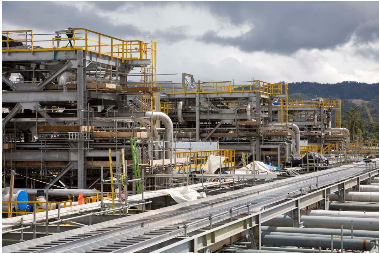
Hides Gas Conditioning Plant, June 2013.
