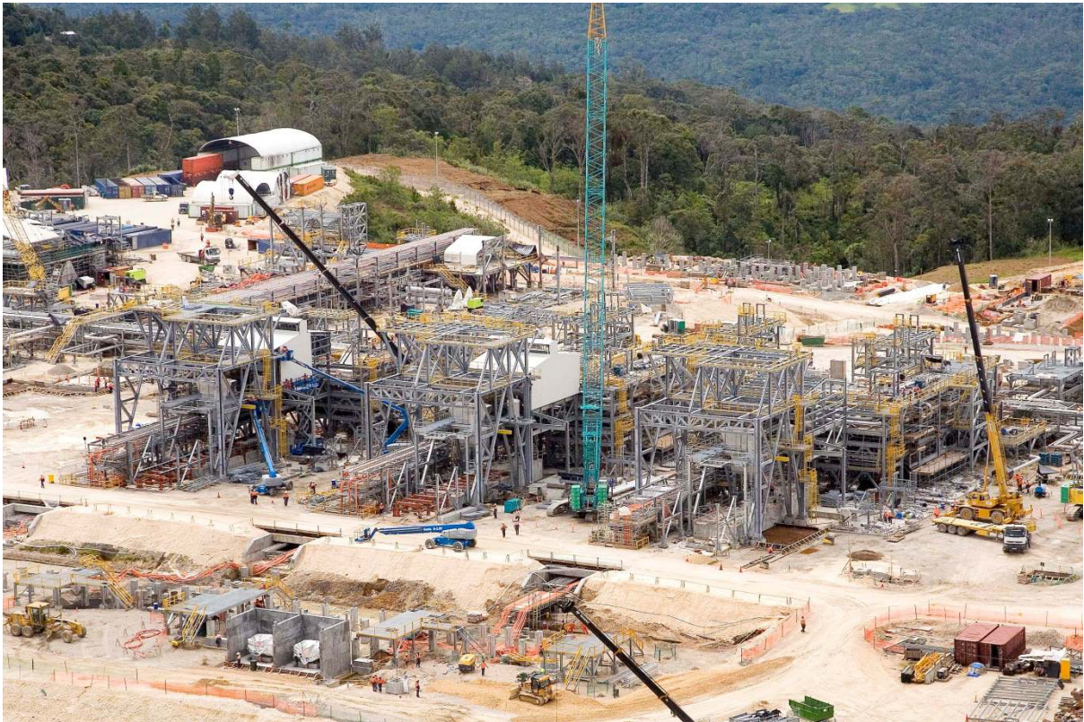
Hides Gas Conditioning Plant, May 2013.
