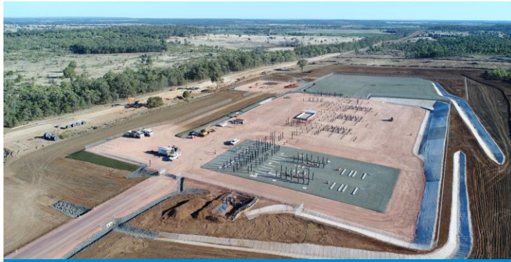
Roma nodal compressor station
