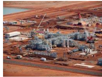
Devil Creek gas plant
