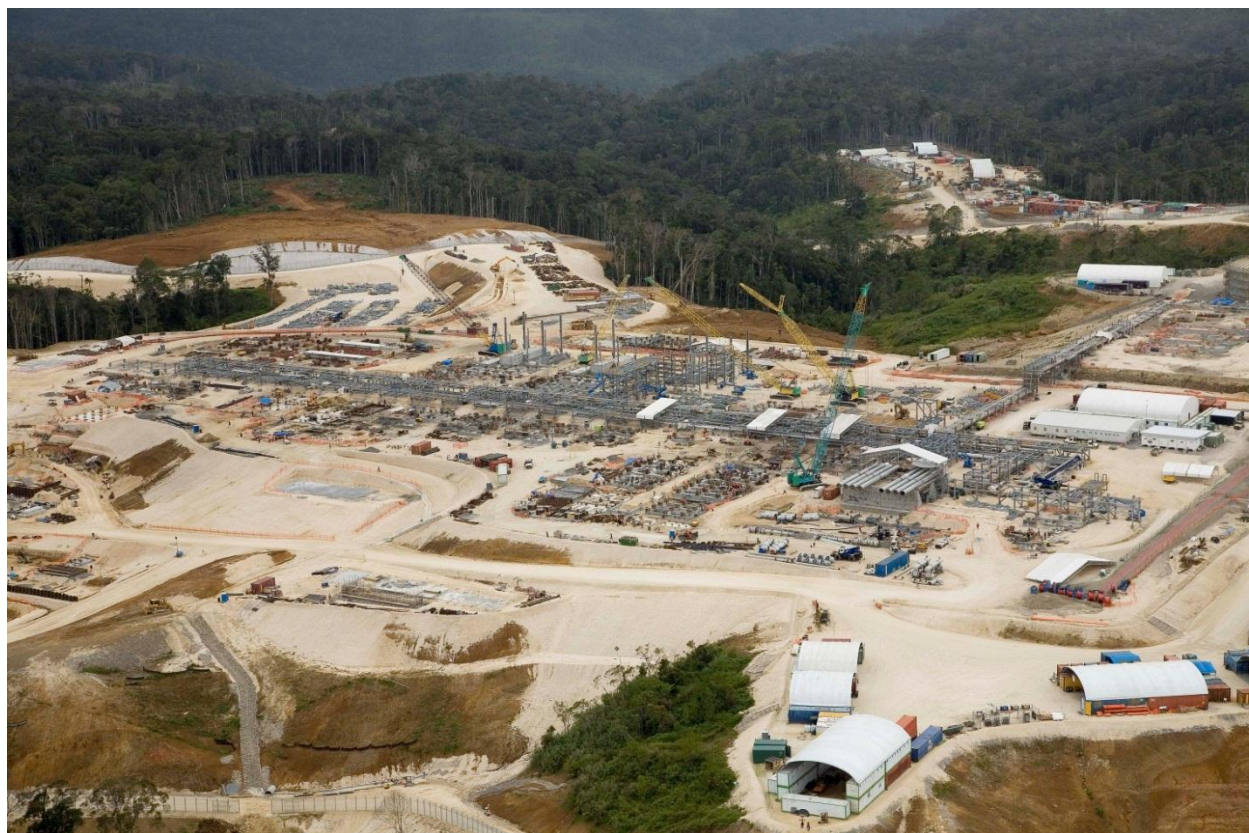
Hides gas conditioning plant, December 2012
