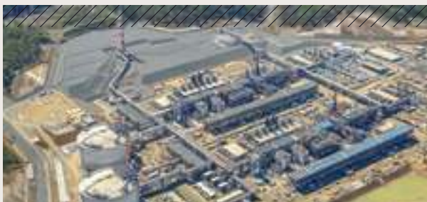
On track for first LNG around the end of September 2015. GLNG plant, Curtis Island, Queensland
