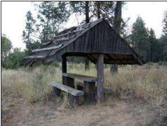
Figure 4.108: Roadside shelter showing damaged roof (Image: ARCHAEO 2008).
