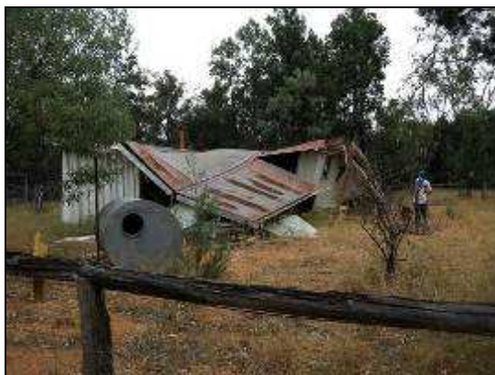
Figure 4.102: Collapsed barracks building (Image: ARCHAEO 2008).
