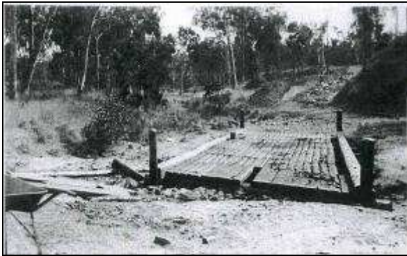
Figure 4.9: Photo of the crossing from the south bank during repairs c.1937 (Image courtesy of the Queensland State Archives).
