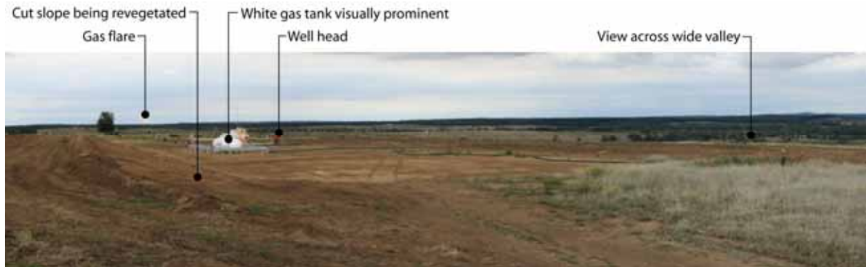
Plate 22 Production well on ridge top with cut and fill slopes prior to revegetation
