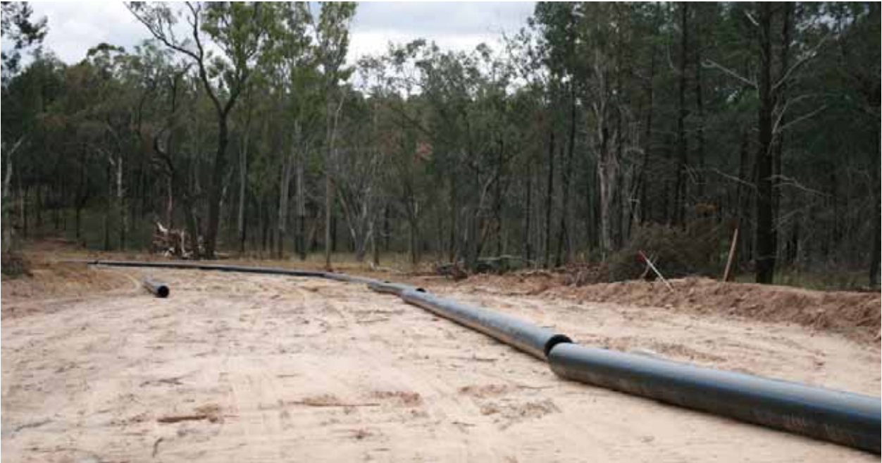
Plate 25 Gas collection pipeline laid out along easement in forest area prior to trenching and installation
