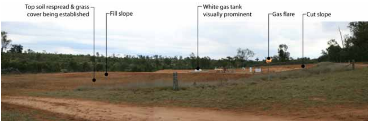
Plate 20 Production well site on undulating landform showing cut and fill slopes prior to revegetation
