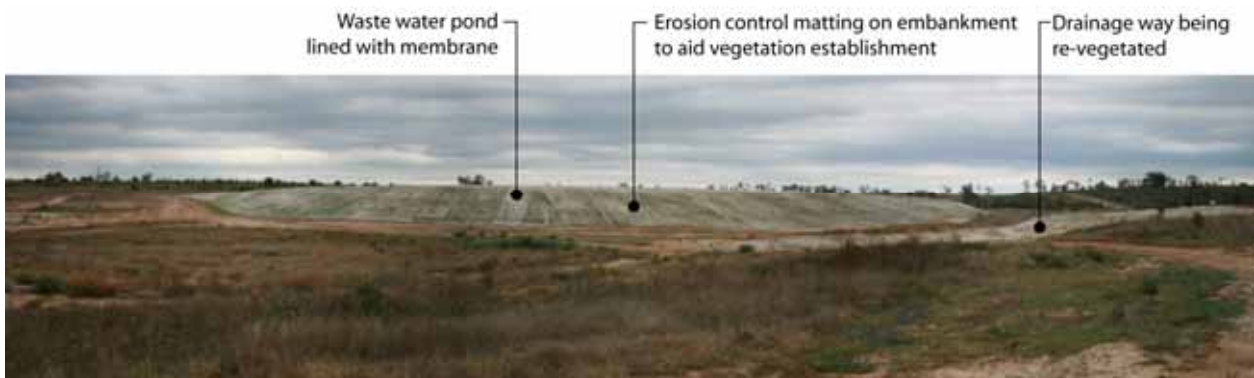
Plate 31 Water storage dam embankment with erosion control matting used to establish a protective grass cover
