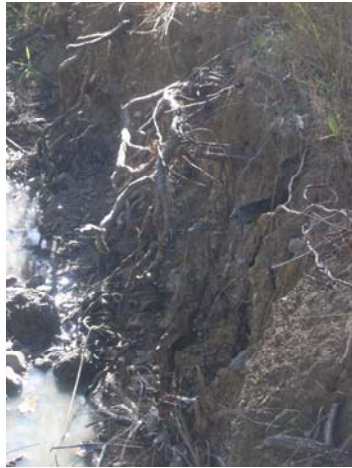
Photo: Eroded left bank
