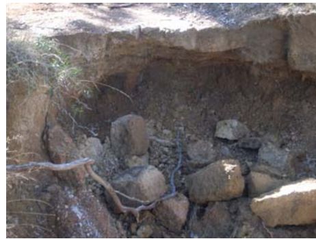
Photo: Undercutting Downstream Bank
