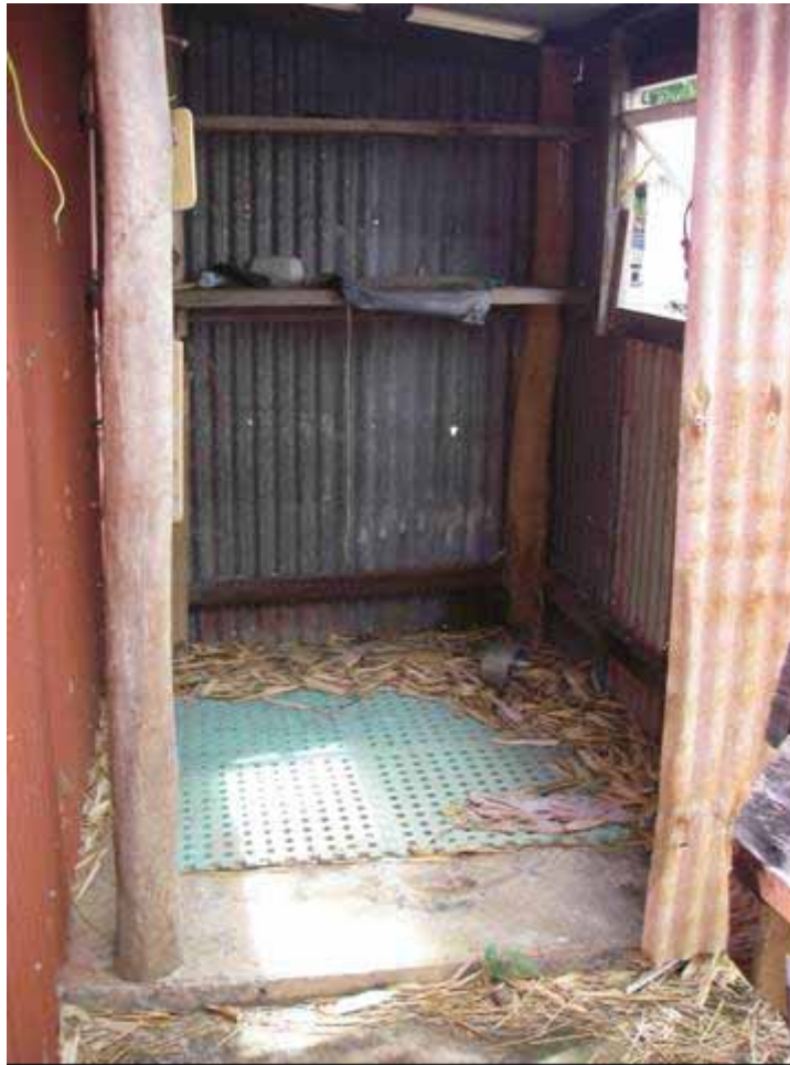
Plate 3-8 Generator shed at Fisherman's Hut
