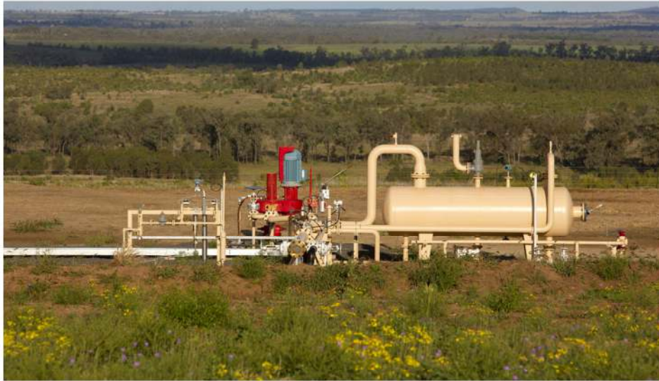
Production well at Coxon Creek, Queensland
